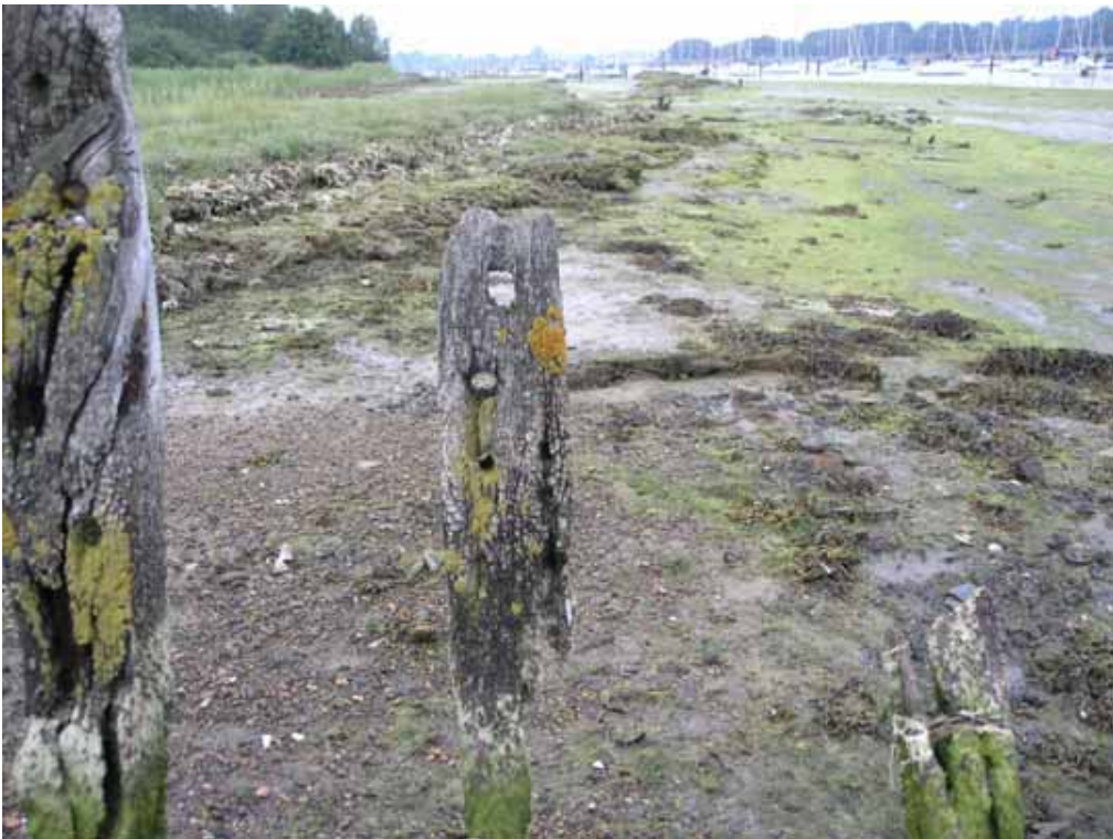
Figure HAM051- 7 The upper part of this frame lies above the high tide and is less eroded than the timber that lies within the tidal range
