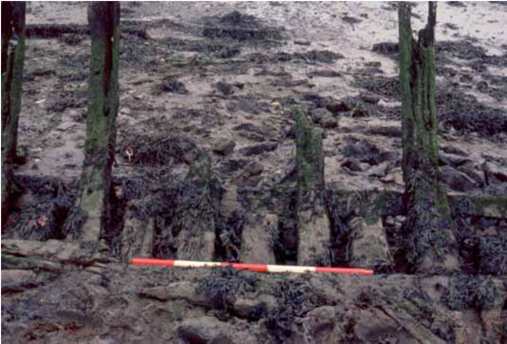
Figure HAM051- 6 The remaining frames have been broken off or eroded to different heights (looking north)
