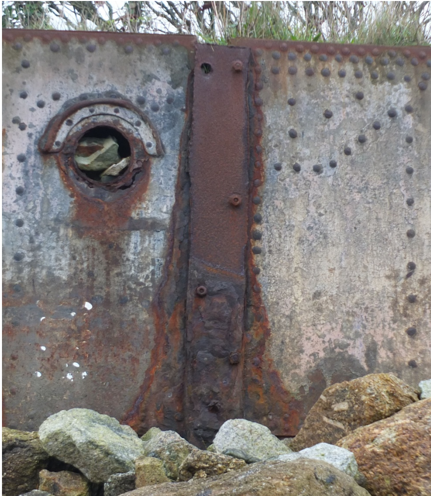
Figure 12: joining strip between panels 6 (left) and 5 (right) – the riveting pattern at the gunwale changes
