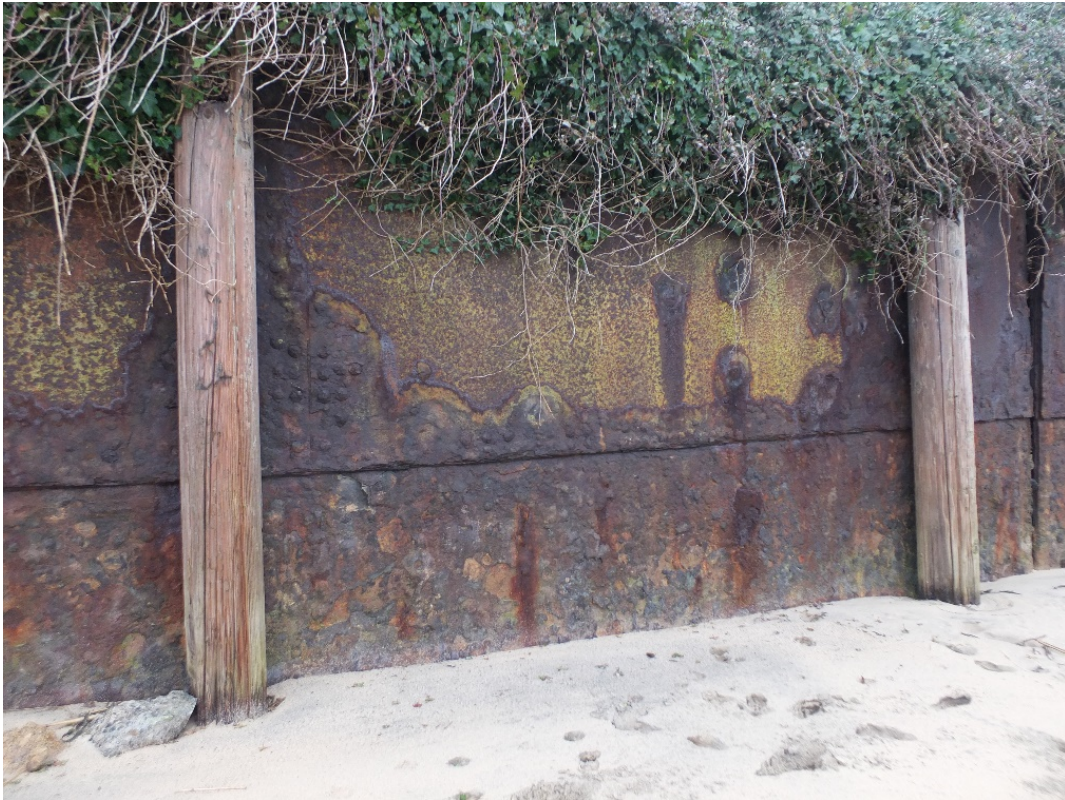
Figure 38: Treble chain riveted vertical butt joins, double riveted horizontal lap joins in Section C
