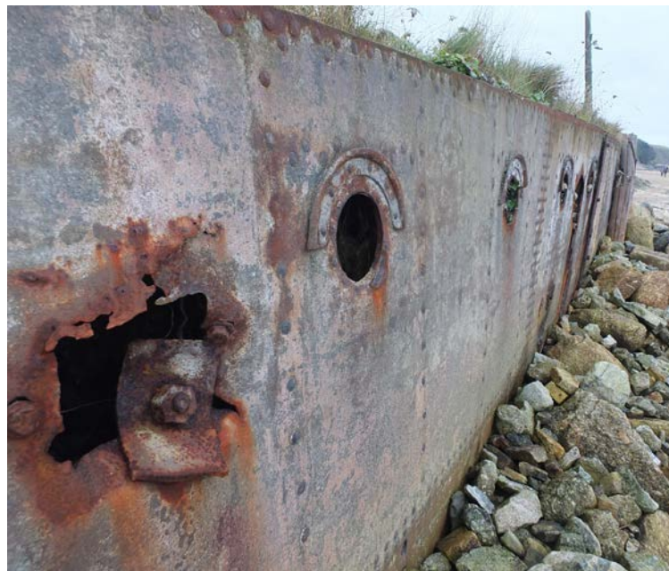
Figure 20: rectangular opening in hull plating, Panel 7
